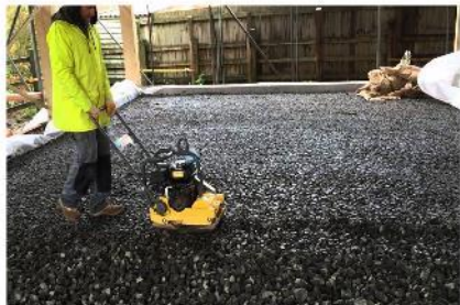
Design to reduce the use of concrete by replacing the slab with Recycled Foamed Glass and Natural Hydraulic Lime Screed. Concrete is minimised to a perimeter ring beam.
